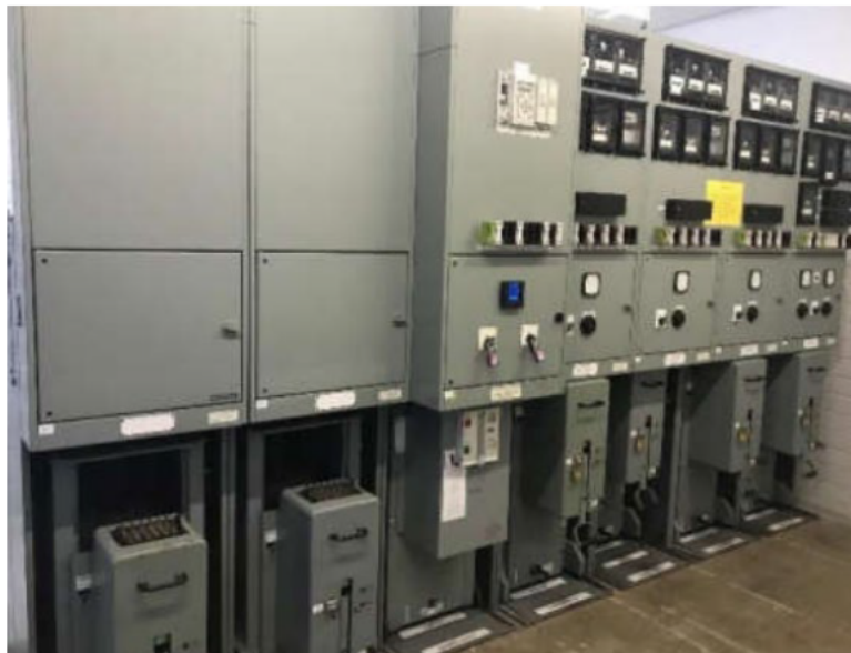
Figure 5 Legacy switchgear (LHS) section at St Fergus
